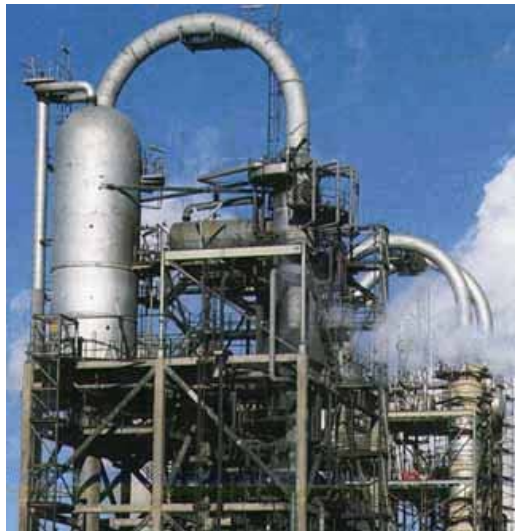
Figure(5) Fluidized-bed Reactors
